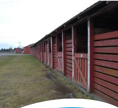
Stalls and barns in the centre of Beban Park are in poor condition.
