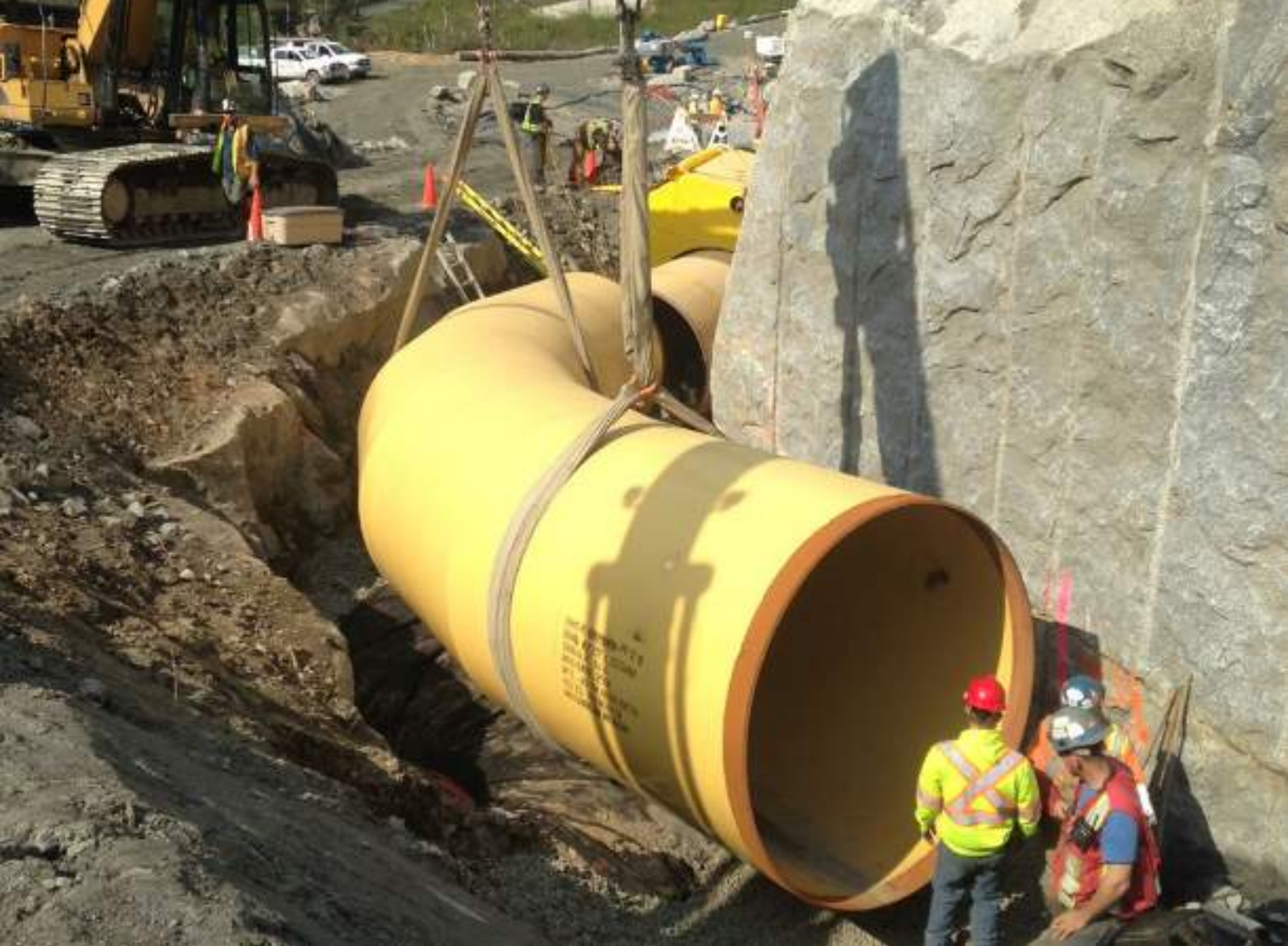
Above: Jimmy Creek Hydro Project, Hazelwood Construction Photo Courtesy of Hazelwood Construction Services
