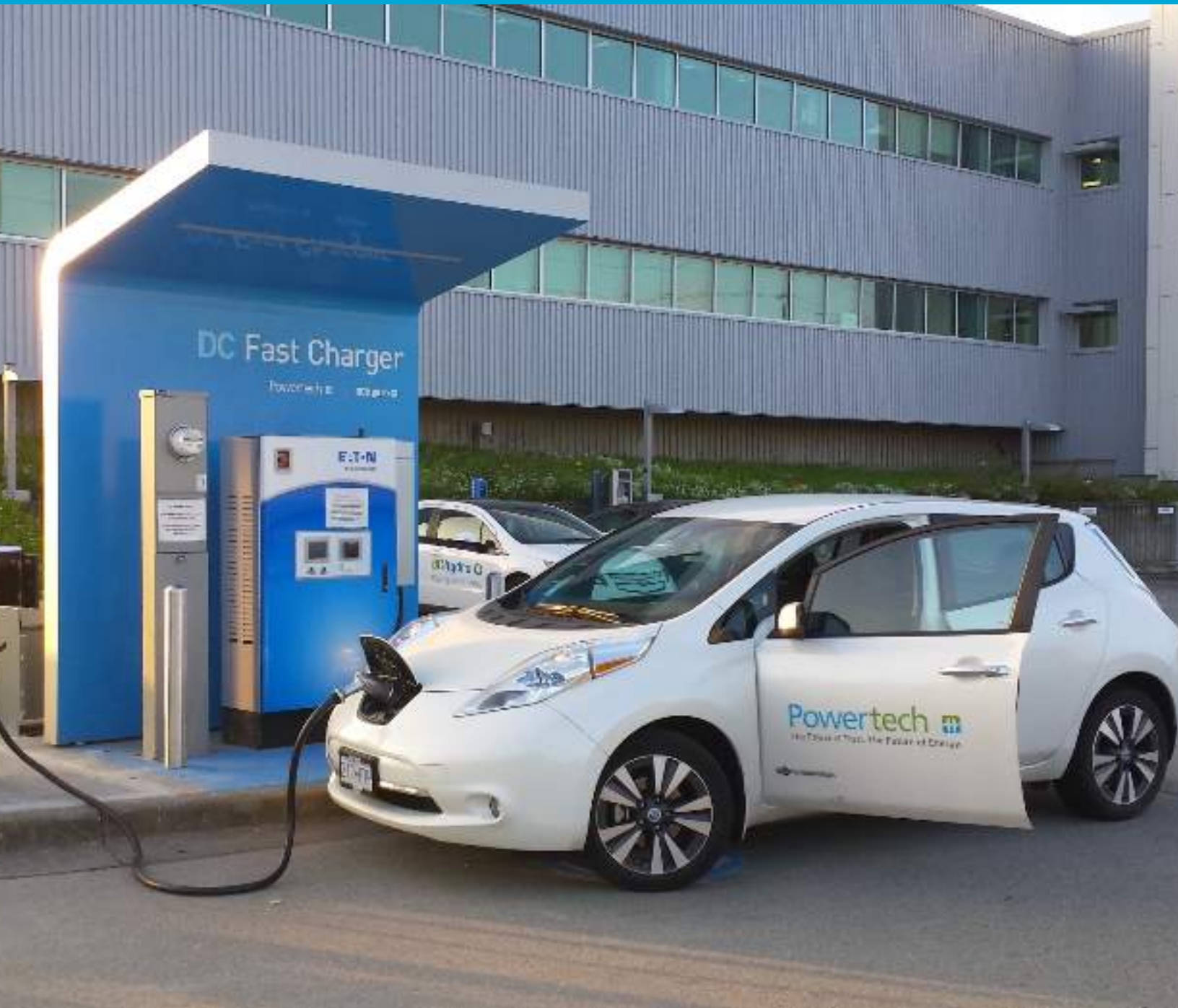
BC Hydro EV Charge Park at Powertech Labs – Multi-DC Fast Charger Station for Advanced Operations Testing
